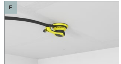
Sand joints: After sanding with preferred tool, ensure that the joints are perfectly smooth.
